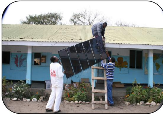
Technicians Installing Solar PV System for a rural Health Centre in Bagamoyo
